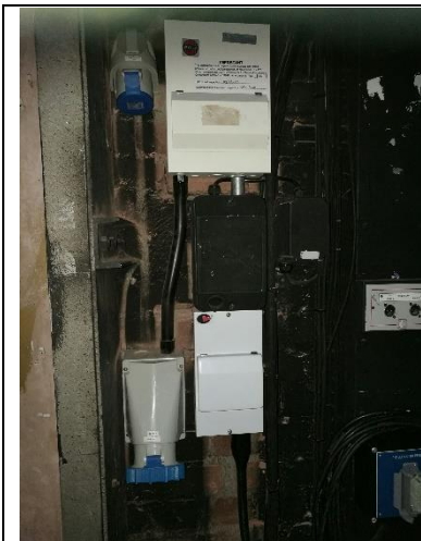
Sound Power single phase 63a 32a located DSR
